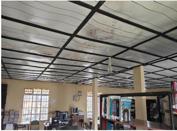
MMTU Goderich Library with identified leakages in the ceiling
