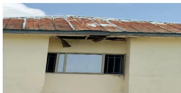
Side View Showing Damaged Ceiling of Admin. Building
