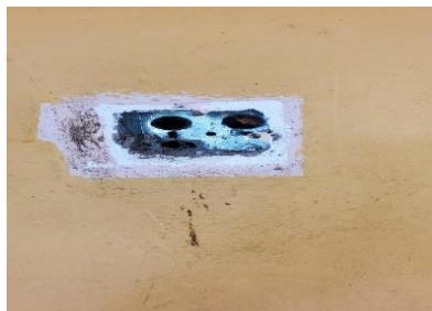
Stolen electrical fittings
